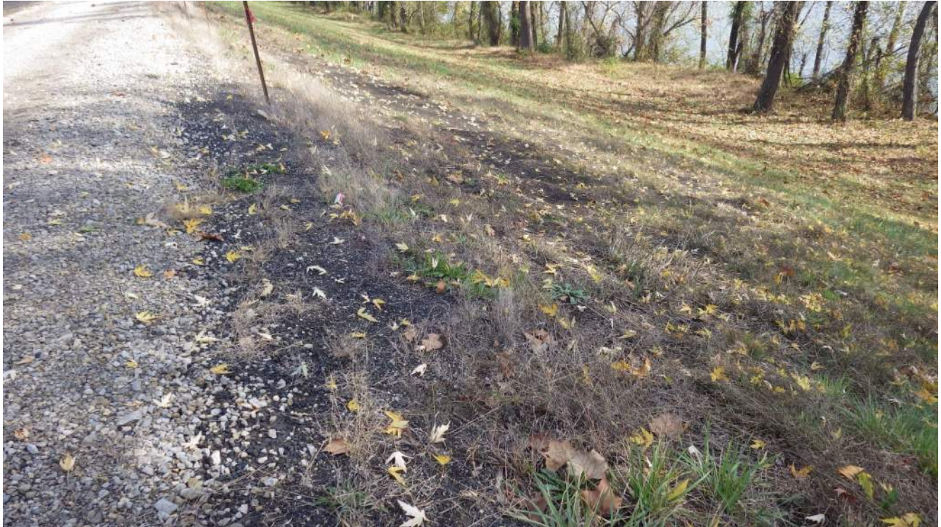
Photograph 15 – Minor erosion of surface material between BSP and Ohio River.
