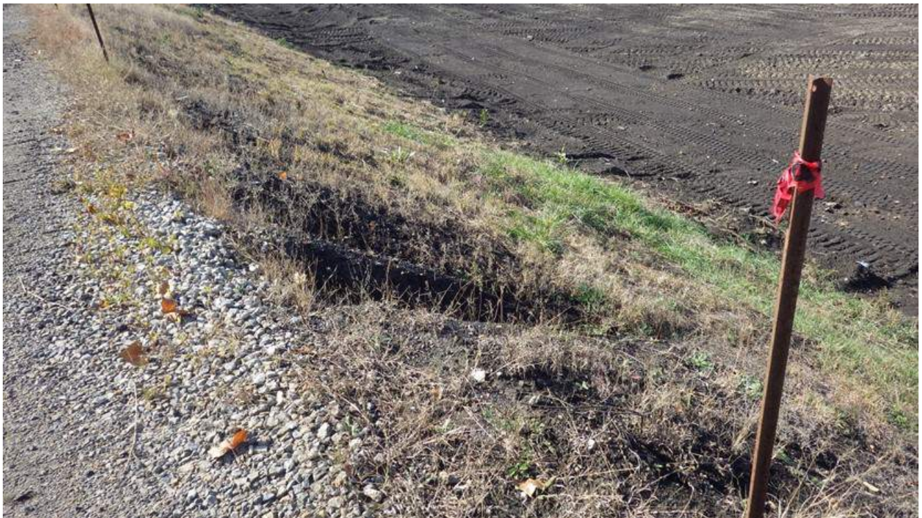
Photograph 16 – Erosion gulleys located on interior dam surface near northeastern corner of BSP.
