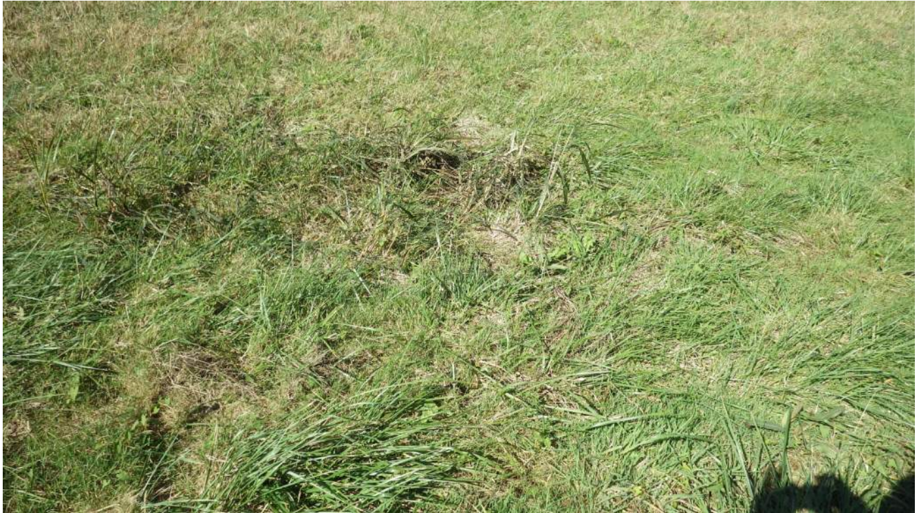
Photograph 7 – Erosion at toe of eastern embankment.
