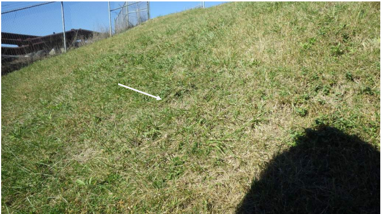
Photograph 4 – Minor surface sloughing of eastern slope of SFAP along State Route 7.
