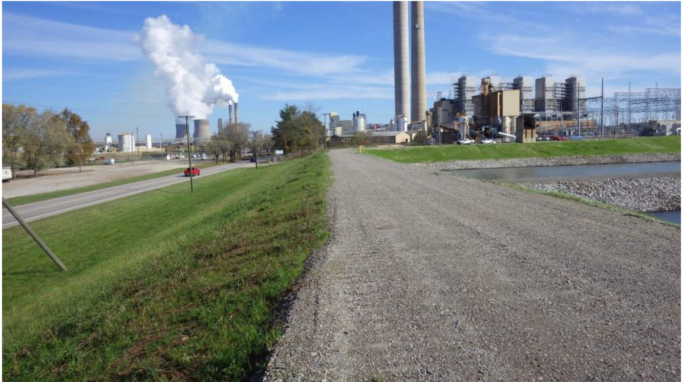
Photograph 5 – Erosion noted at change from access road to grassed slope.
