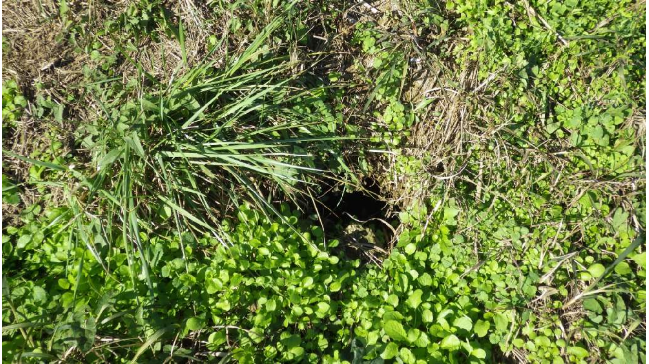
Photograph 9 – Small hole on eastern downstream slope of SFAP.
